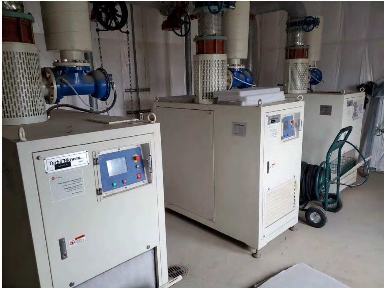
Figure 3-8: Existing Neuros Blowers in Blower Building
