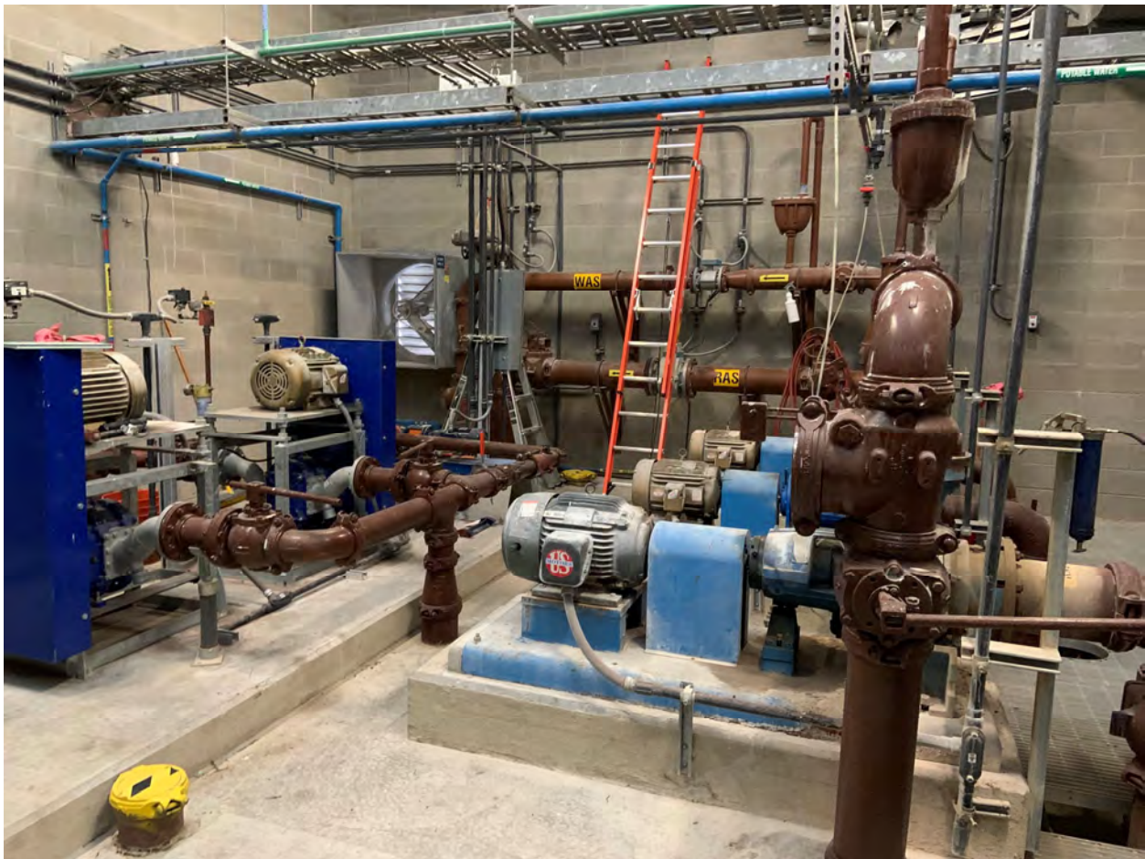
Figure 3-14: RAS/WAS Pump Station in Biosolids Building
