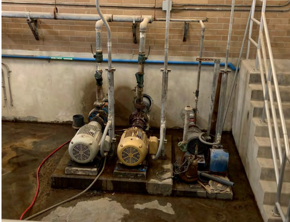
Figure 3-17: Utility Water Pumps
