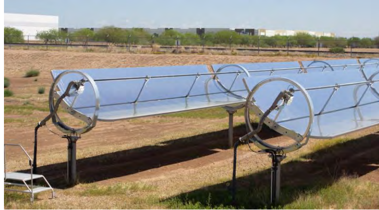
Figure 3 - Parabolic trough solar thermal collectors
