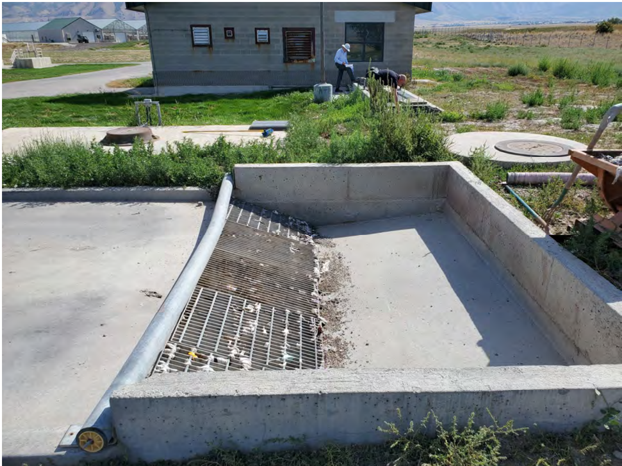
Figure 3-2: Septage Receiving Station
