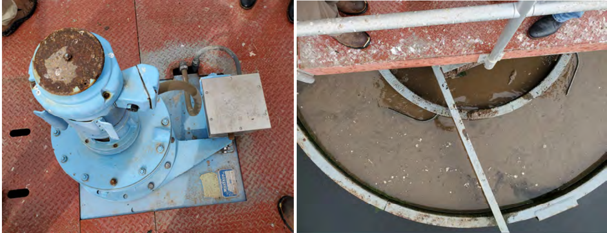
Figure 3-12: Drive Assembly and Feedwell of Clarifier #2
